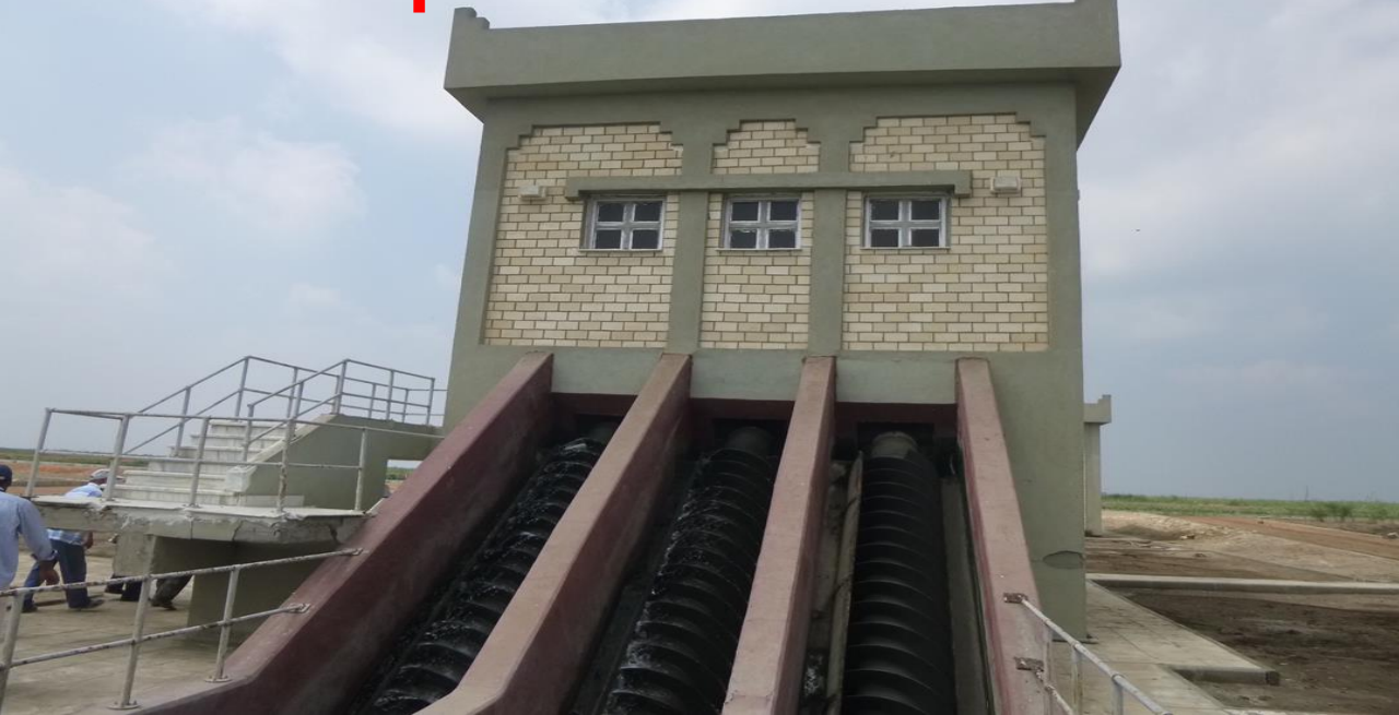
Pump Station on Drain
